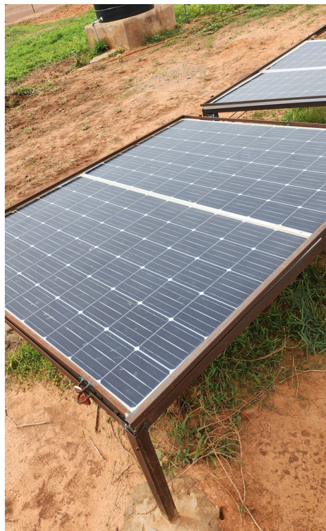
Solar Powered Borehole
